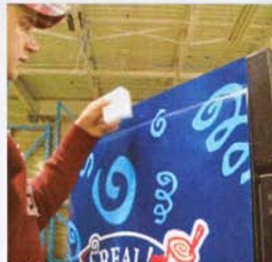
Step 3 From right to left begin squeegeeing decal to freezer. Press firm to apply properly.
